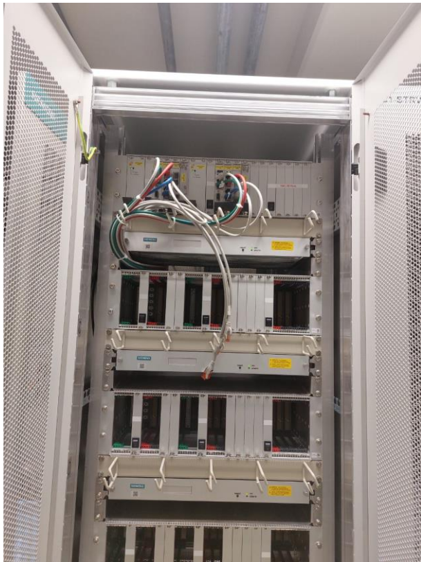
Innenanlage: Radio Block Center
